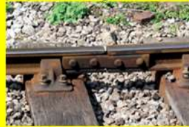
Figure 5: The gaps along railway tracks
